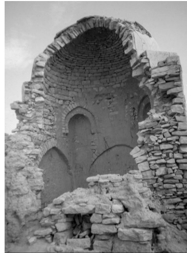
Fig. 5 - Barāqish. The chahār ṭāq mausoleum, west half: the interior, showing walled-up doorways, squinches and the dome (© M.V. Fontana 1992).
