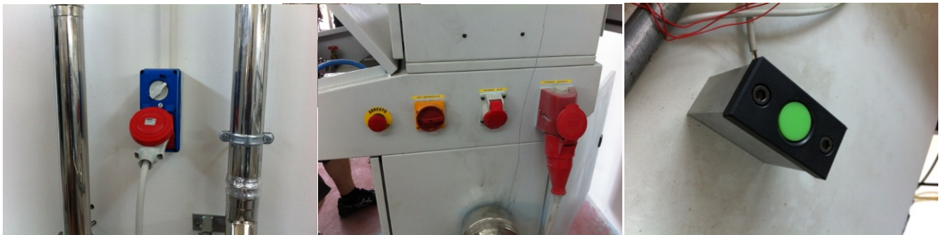
Figure 8. Compressor air supply and test bench switches Ignition button.
