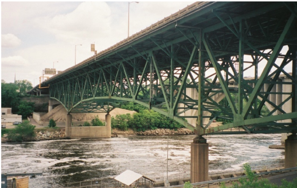
Figure 7.1. I-35W Bridge [NTSB, 2008].
