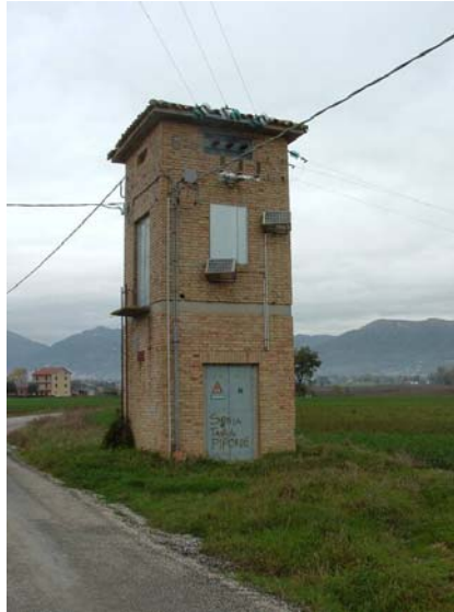
Figure 3.7. ENEL electrical substation housing a recording instrument in Gubbio-Piana site (Umbria)
