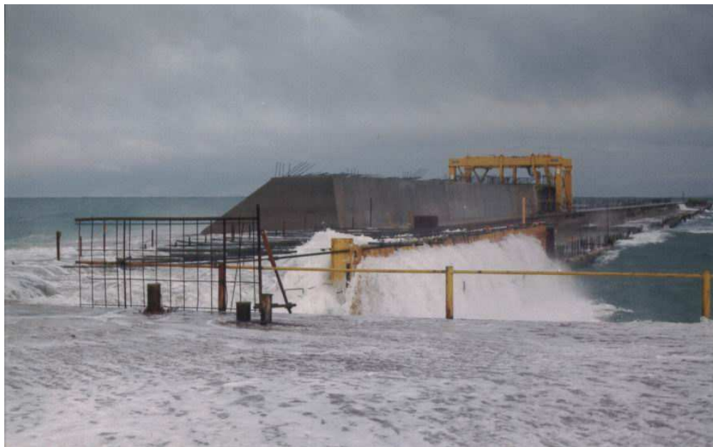
Figure 28. Construction of superstructure (II Extension) under the storm of 23 rd February 2004 (photo's Pietro Cidonio S.p.A)
