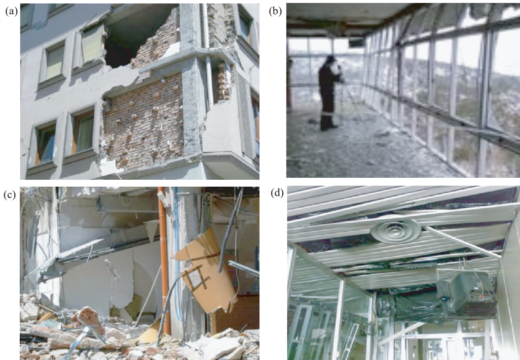
Figure 1.4. Examples of deformation-sensitive nonstructural components and their damage. (a) External cladding panels. (b) Glazing. (c) Interior partitions. (d) Suspended ceiling. After Dipartimento della Protezione Civile [27].
