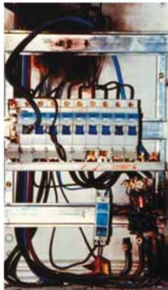
Figure 4.1. Low-voltage switch board without SPD singed due to lightning overvoltage [90].
