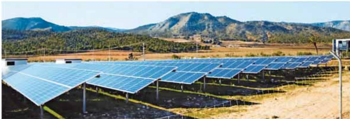
Figure 8.8. Industrial photovoltaic power generating system [204].
