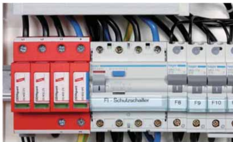
Figure 4.2. SPD installed in low-voltage switch board [90].
