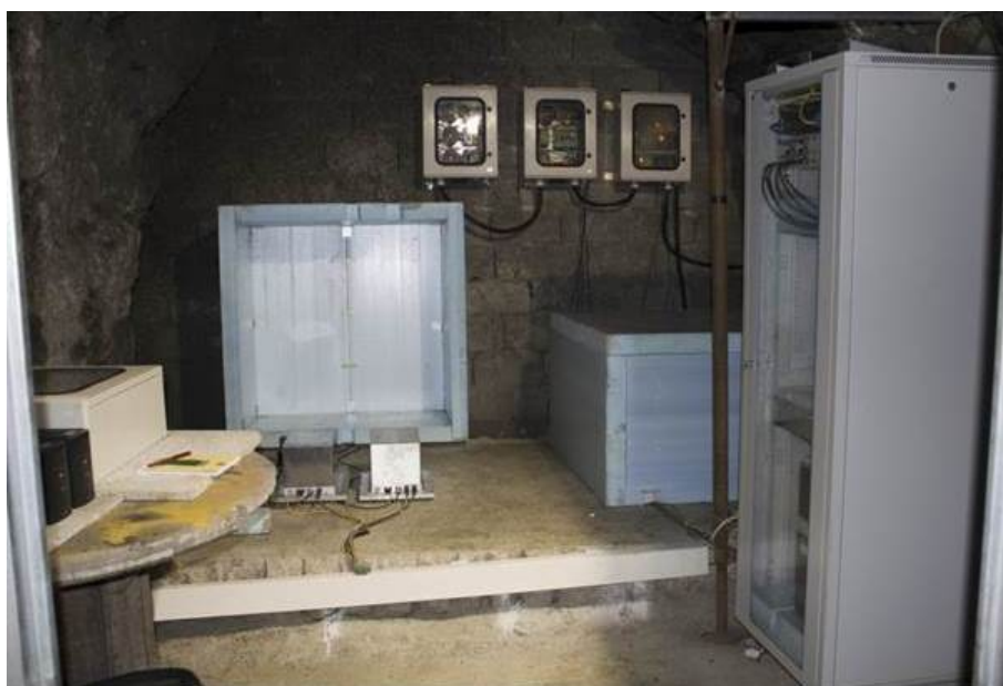
Figure 5.11: The underground station -1. The horizontal seismometers built at the university of Salerno [140] are placed on a plinth cemented to the bedrock, and enclosed into insulation boxes (one opened in the left, the other closed in the right).
