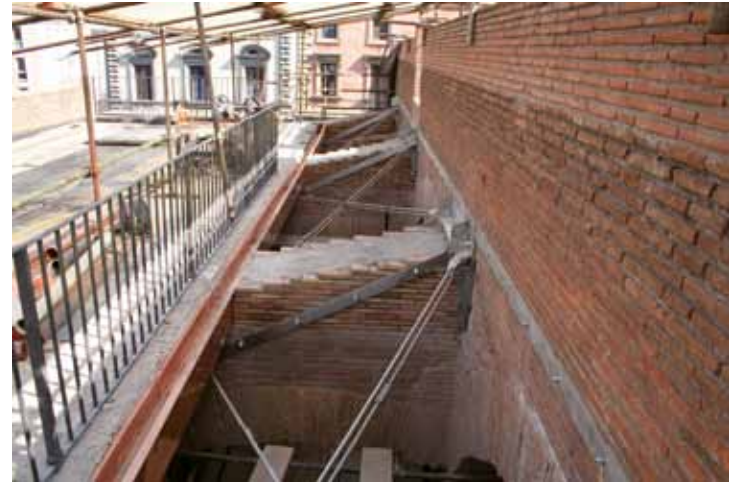
Fig. 11. View of the southern lateral longer side of the Great Vault with the diagonally counterbraced shear reinforcements placed in the free spaces between the Vault itself and the Southern building, nearly the ending of the work.
