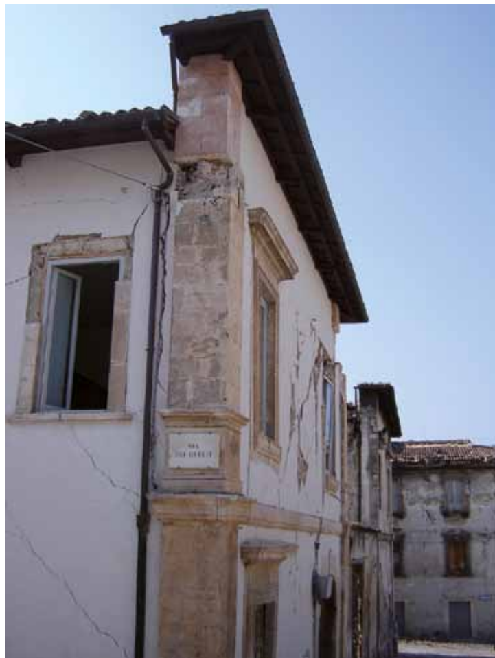
Fig. 3. L'Aquila. Shear cracks on the external walls of a building that confirm the box behavior of the masonry assembly.
