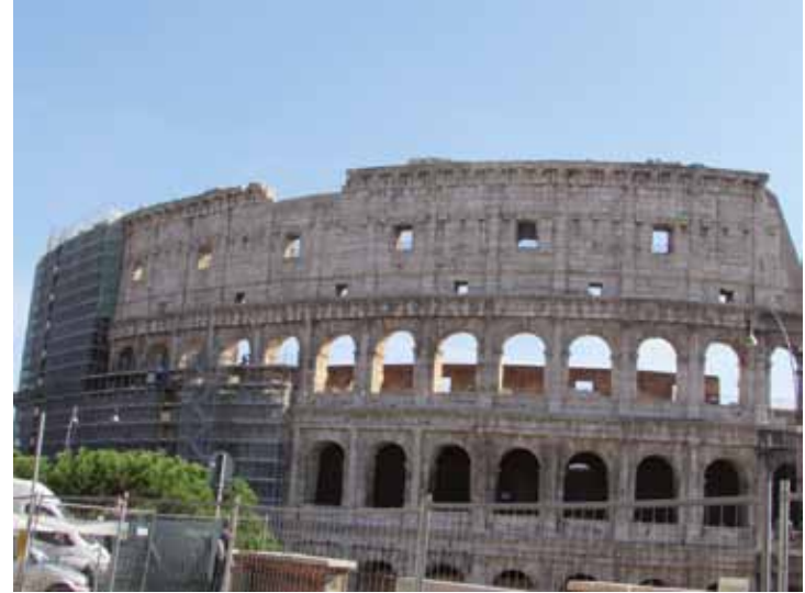
Fig. 8. Coliseum, Rome (Italy): Façade North, dismantling and assembling the scaffolding (ph. B5 srl).
