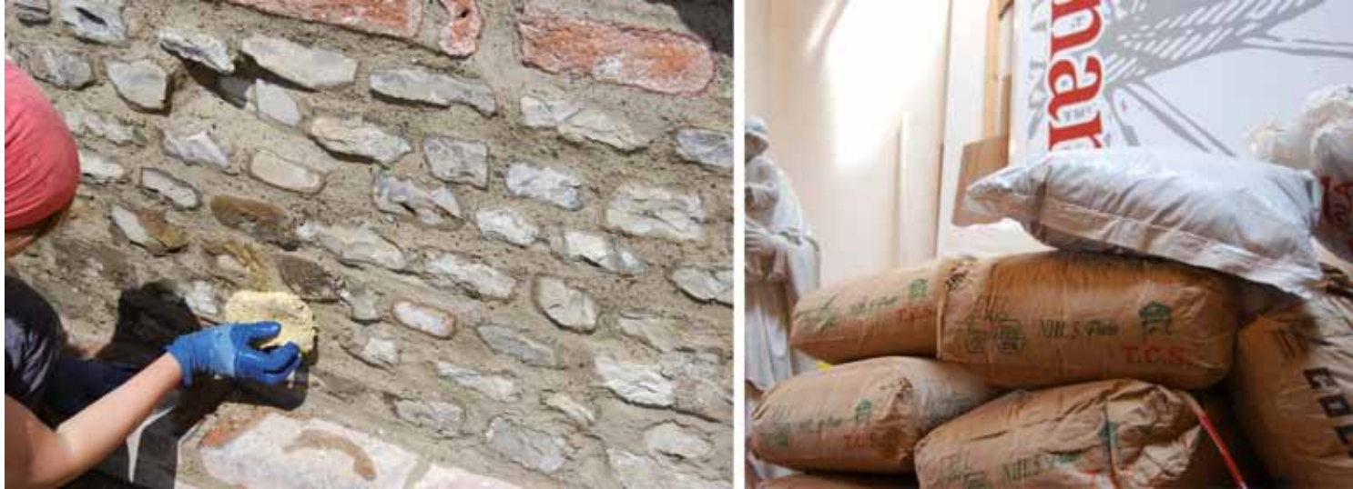
Fig. 3. Use of mortars made ad hoc in analogy with the original materials.
