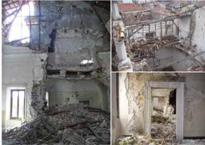
Fig. 1. Views of some collapses: a wall in the main hall of the palace (with the light vault), the loggia over the roof and the rooms in the main floor.
