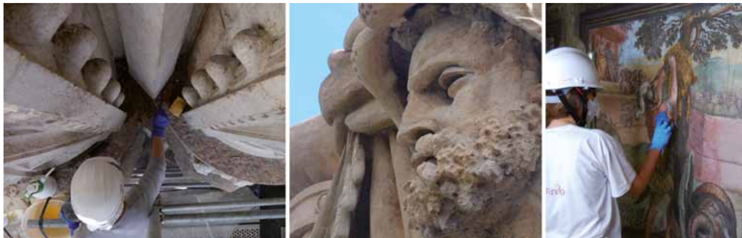
Fig. 2. Interventions carried out on the Basilica of San Petronio, Palazzo Fava and Villa Hercolani, Bologna.
