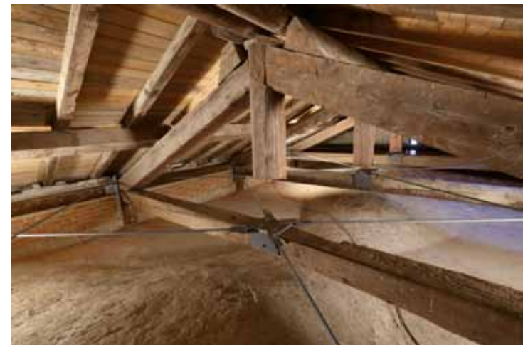
Figs. 8-9. The restoration and strengthening of wooden structure of the roof and of the upper perimetrical masonry in the area of the museum.
