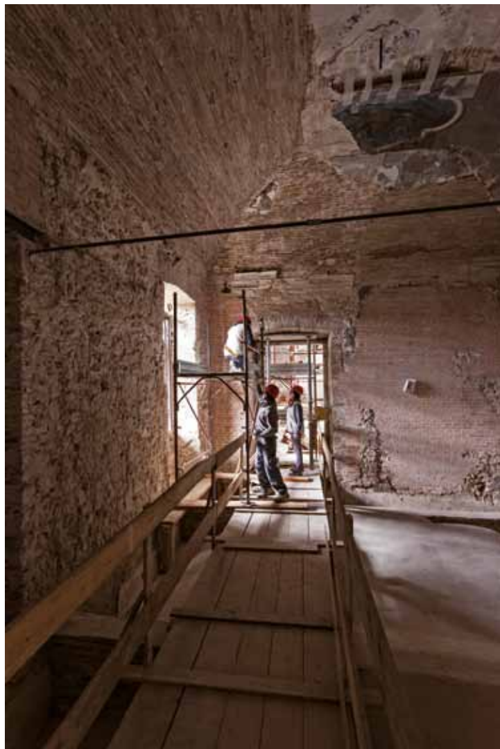
Fig. 5. Work into a room of the building, with the integration of the wall with cuci-scuci system.
