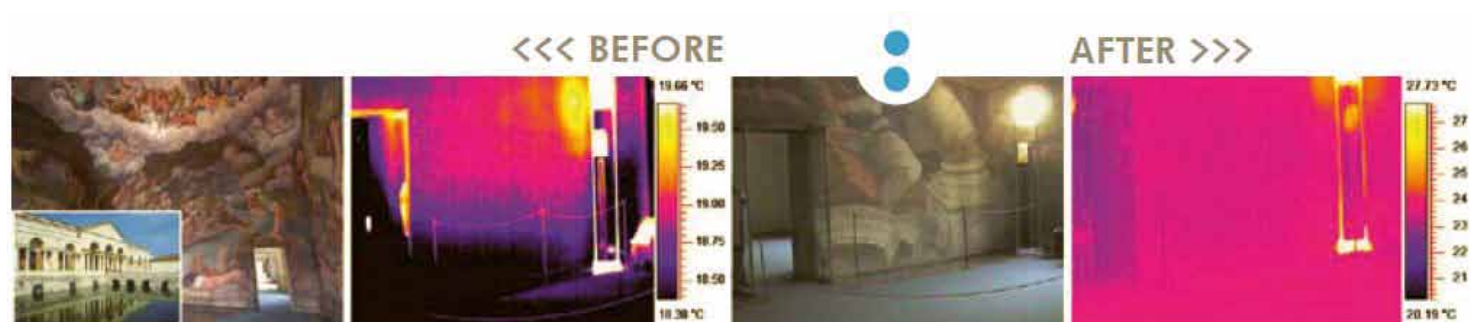
Fig. 3. Mantua - Palazzo Te, Hall of the Giants. System installed: no. 2 Domodry® LS-R15 units.
