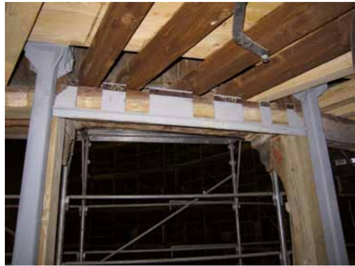
Figs. 6-7. Detail of the steel strengthening structure that allowed the preservation of the original wooden. After the end of the restoration it will be completely invisible, not to modify the overall look of the hall.
