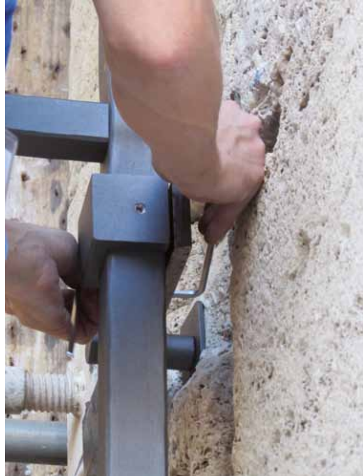
Fig. 6. Coliseum, Rome (Italy): Low impact system of fixing new gates (ph. B5 srl).
