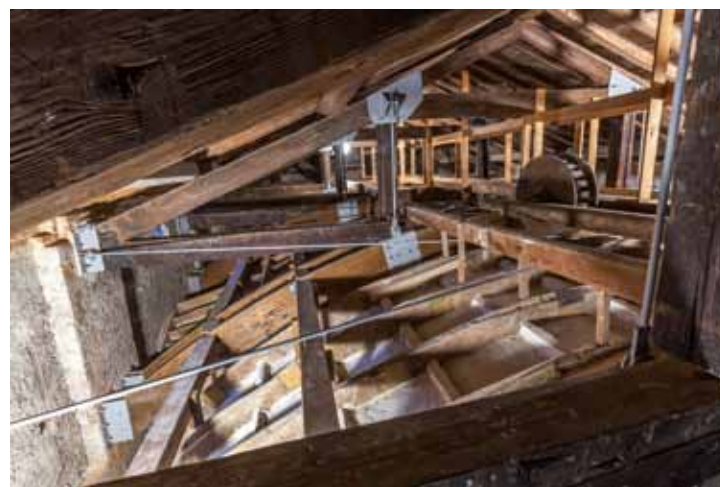
Fig. 13. Detail of the reinforcement of the roof and of the ceiling thanks to metal joints and tie-rods.
