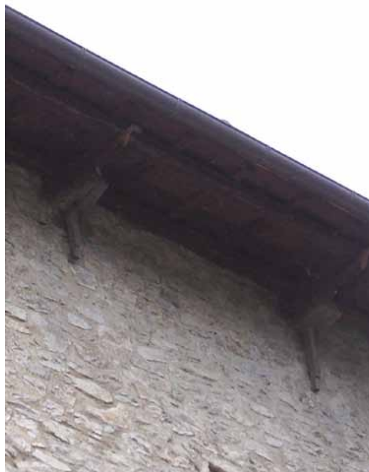
Fig. 2. Paganica (AQ). Tie-beams of the roof trusses of a church's nave systematically anchored to the side walls with wooden pegs ( impalettature ).
