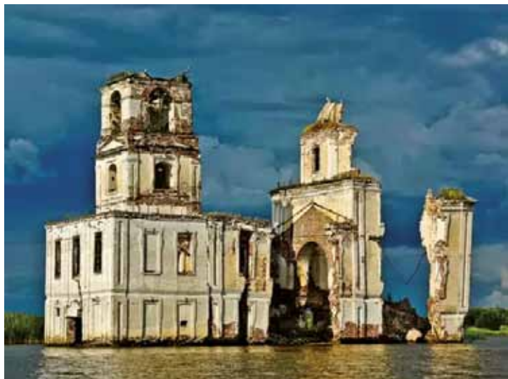
Fig. 1. Church 1, the end of the 18 th century, settlement of Krokfino (Vologda Region) In 1964 was saved from demolition by hydraulic engineers. The church retained all the structures then but later on it was driven to a critical alarm condition by local plunderers.
