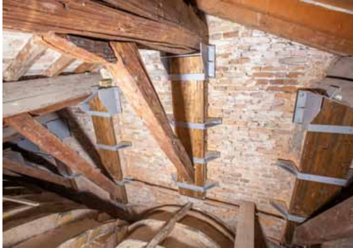
Fig. 7. The reinforcement of the wooden structure of the roof of the monumental stairway, with the new metal and wooden elements connected to the masonries.
