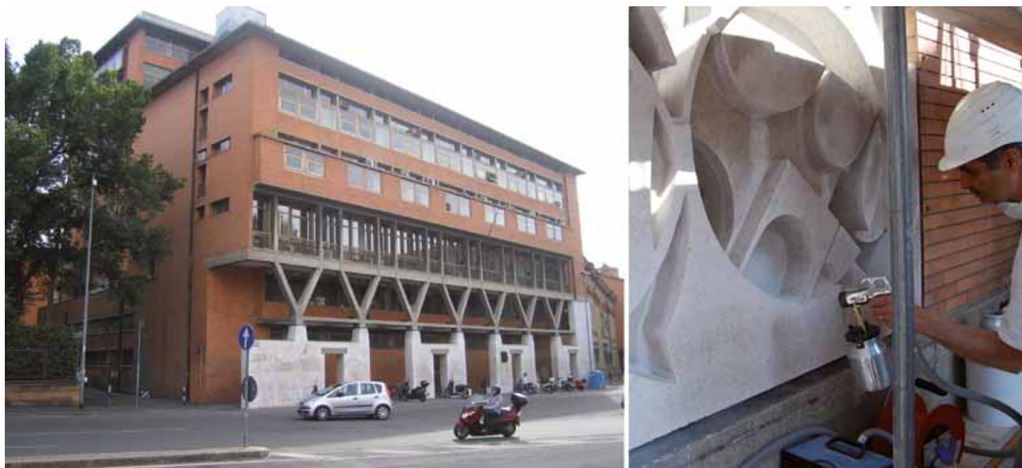
Fig. 7. Coating with photocatalytic protective at the Faculty of Mathematics, University of Bologna.
