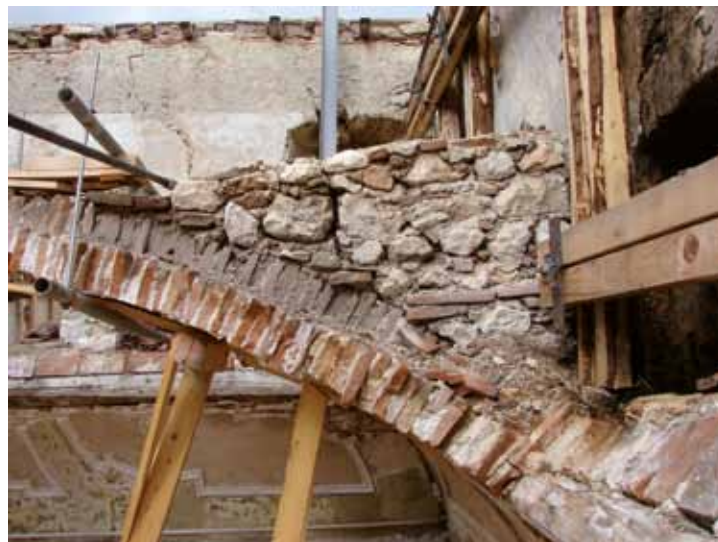
Fig. 5. L'Aquila. Wooden tie-rods at the springing of the coves in a cloister vault in Palazzo Ardinghelli.
