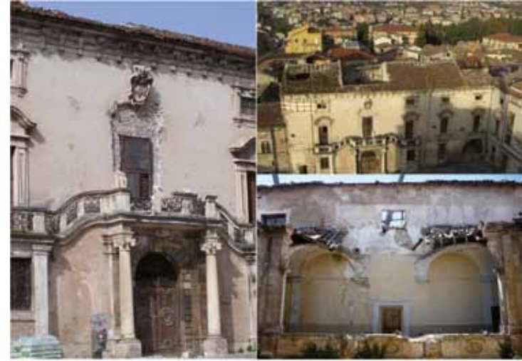
Fig. 2. Views of some damage: the main façade, the roof, the corridor in the inner courtyard.
