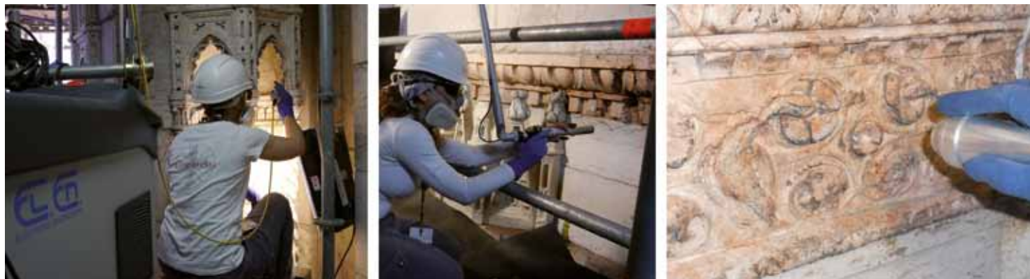
Fig. 5. Cleaning with laser system on the stone facade of the Basilica of San Petronio.
