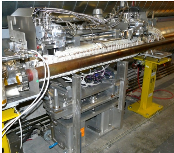
Figure 5-3: Photograph of the active absorber TCLA.B6R7.B1 as installed in the betatron cleaning insertion.
