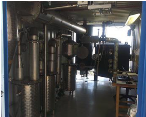
Fig. 2. Picture of the plant in the skid.
