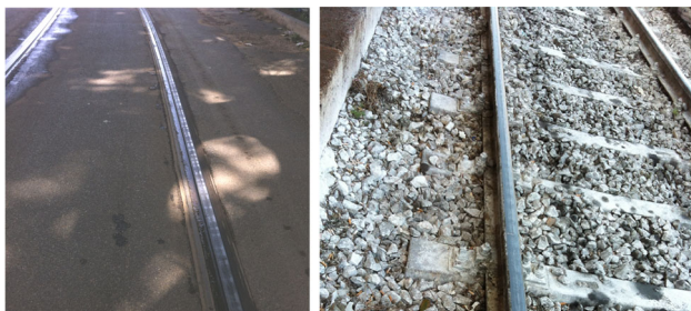
Fig. 5 Wear on tramway and railway tracks
