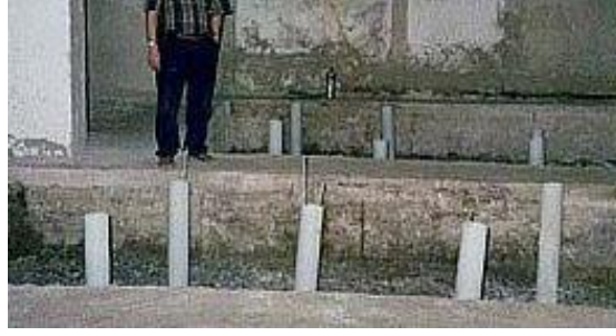
Figure 4. Vertical drains installed in the foundation soils of the building during construction works (Sezer, 2020)
