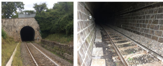
Figure 10. Galleria Sipicciano I: Photo of tunnel entrance ch. 7+228 (on the left) and photo inside the tunnel (on the right).
