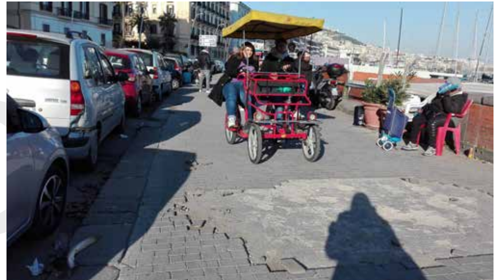
Fig. 2. Some vulnerabilities along the waterfront pavement of Via Caracciolo: damages (broken/missing slabs), rickshaw and scooters, waste and cumbersome objects (Cuturi C., February 2023).
