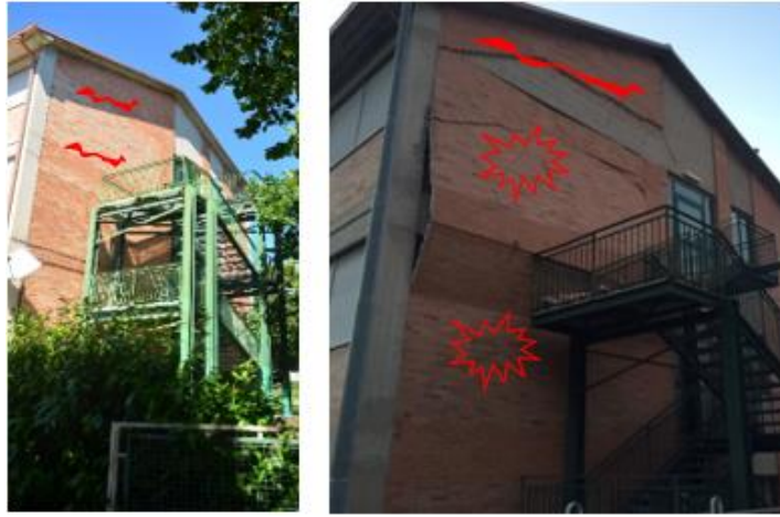
Figure 15. Damage state on the external infill after E_a (left) and E_o (right)
