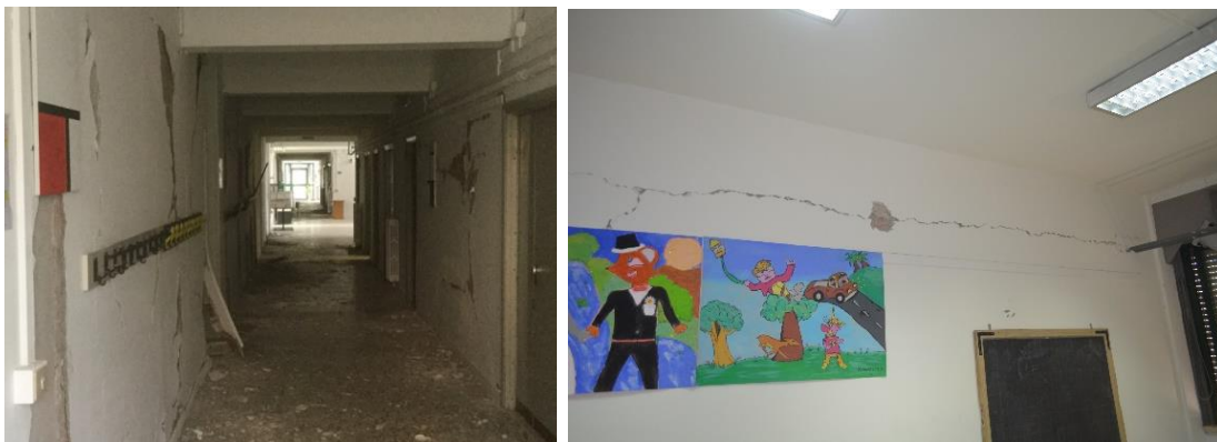
Figure 17. Damage state on the internal infill after E_a (up) and E_o (bottom)
