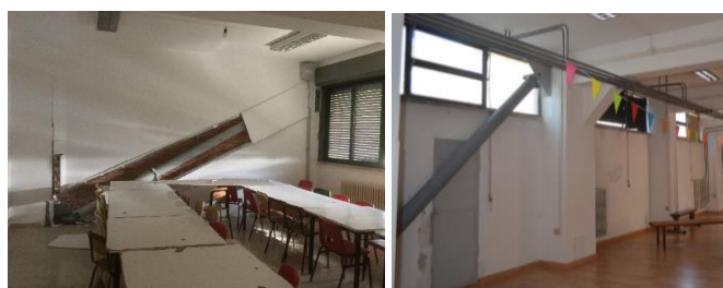
Figure 8. Dissipative device BRAD 14/40-b installed in the building
