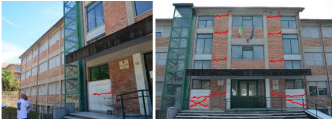
Figure 16. Damage state on the external infill after E_a (left) and E_o (right)
