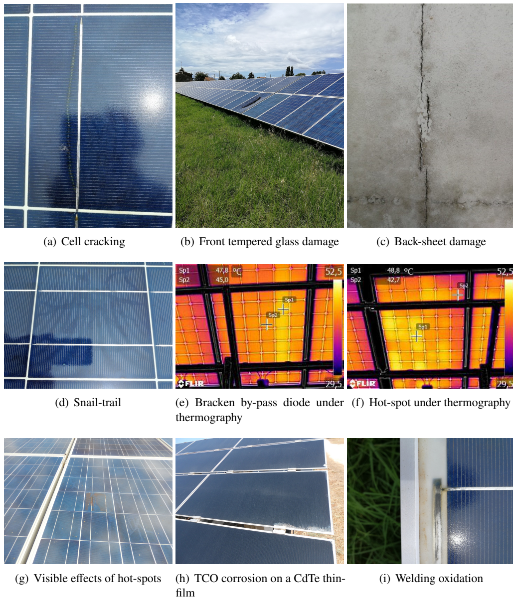
Figure 5.9. PV modules failure.
