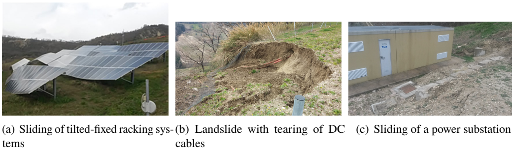
Figure 5.2. Observed slope sliding phenomena.
