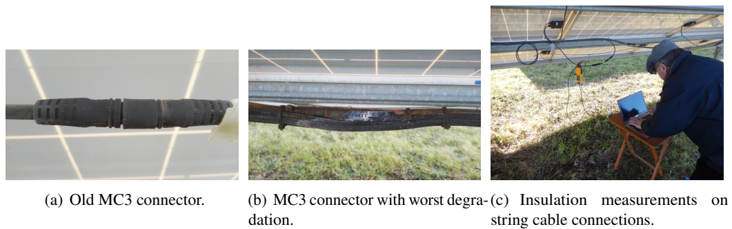
Figure 5.7. Low DC insulation problems.
