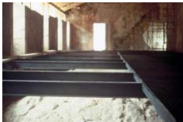
Fig. 20. New beams anchors in the vaults of the Refectory, San Pedro de Arlanza, Salvador Pérez Arroyo and Susana Mora. Photo by Susana Mora, Burgos, 2012.
