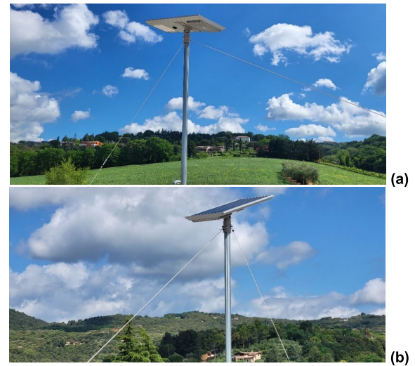
FIGURE 2. View of the solar streetlamp installed in the experimental site: a) from the bottom view of the LED lamp; b) from the top, view of the PV panel.
