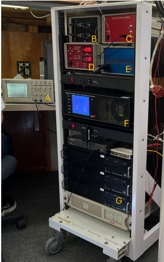
Figure 35 MSO Electronic Controls : A) oscilloscope for fine-tracking quad diode alignment; B) DT drivers; C) dome power; D) camera mount control with x, y, z axis motorized control; E) power box for camera mount control; F) PTC10 unit for MOF and Ws heating; G) computers for dome, MSO-K and MSO-Na control.
