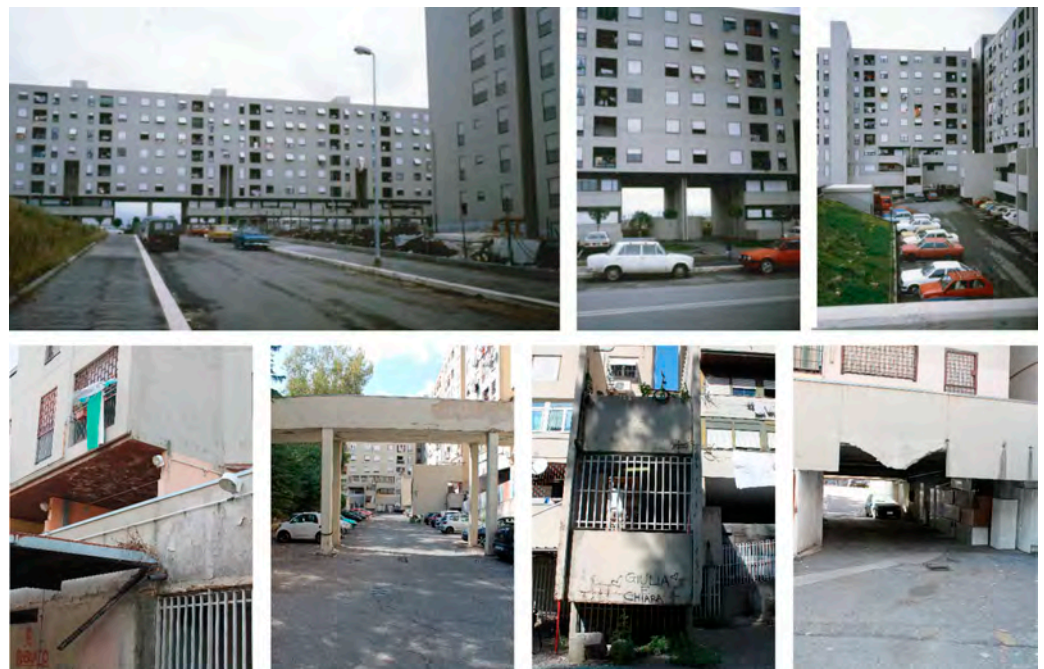
Figure 8. (Top) Images of the neighbourhood in 1983, shortly after completion [30]. (Bottom) Images depicting the current conditions of the compartment R5. The structures are clearly in a critical situation and technological deterioration is evident.
