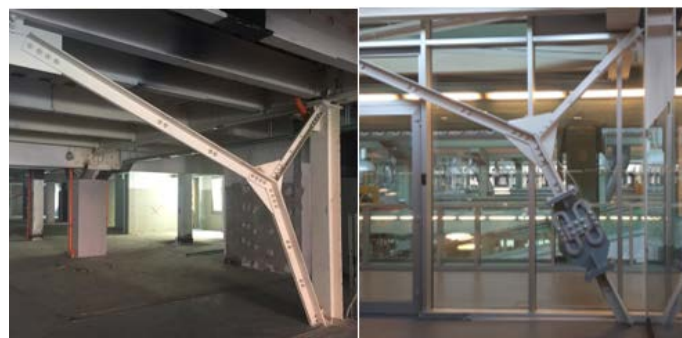
Figure 11. Officine Minganti shopping center (Italy). Bracing before and after the insertion of the HBF dissipative elements.
