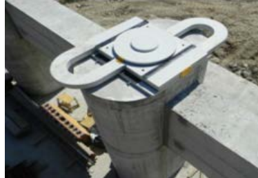
Figure 6. Ingotte Viaduct (Italy) consisting of 4 continuous steel concrete spans. Three AIOS were placed on the central pier and 3x4 longitudinal pot bearings were placed on the abutments and the two lateral piers.
