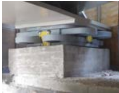
Figure 7. Quadrilatero Marche-Umbria viaducts (Italy). An example of a pair of AIOS working along two orthogonal directions. The project involves the construction of numerous viaducts, all seismically protected with isolators or elastoplastic devices.
