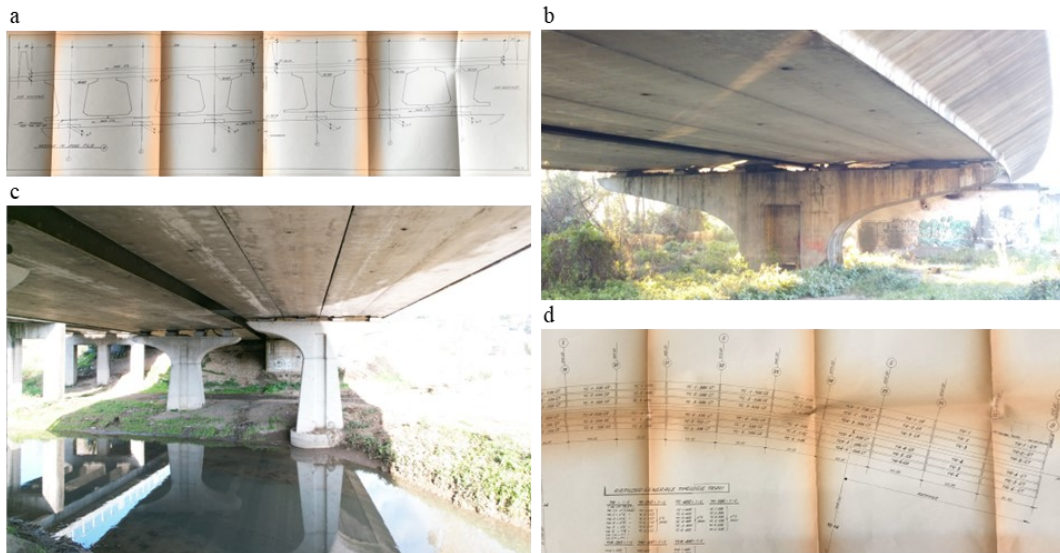
Fig. 1 Case-study: (a) typical cross-section of the deck; panoramic view of a span supported by (b) single piers and (c) pairs of piers; (d) partial longitudinal view of the viaduct.
