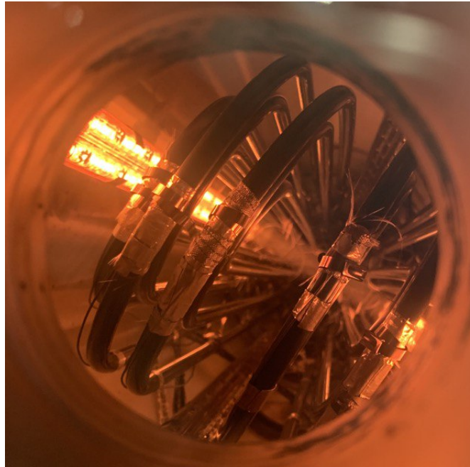
Figure 5.8. Picture of the niobium tubes from the porthole installed on the top of the PAV vessel. The lamps are on and illuminate the tube bundle.
