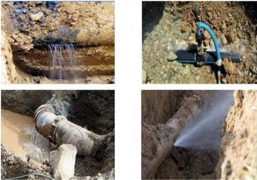
Fig. 2 Several examples of the most common urban water network events in Zanjan city (Water and Sewerage Organization of Zanjan)
