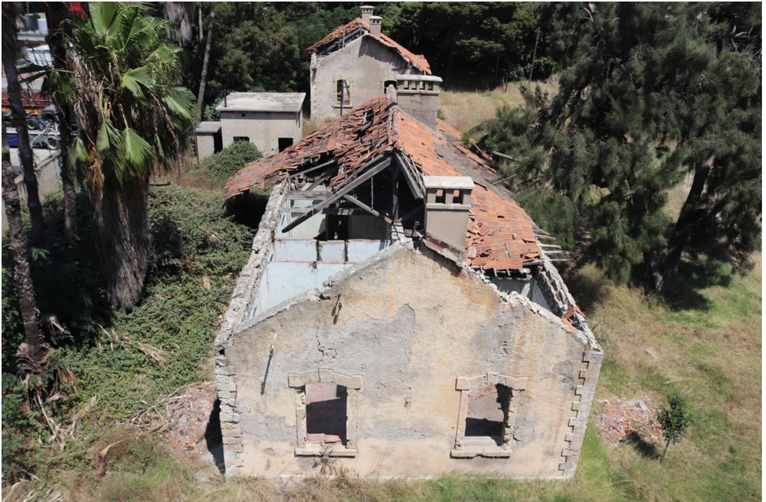
View from historic Memlouki Borj El-Sibai: Overlooking abandoned residences for engineers and high-ranking staff (photo by Yara Rizk)
