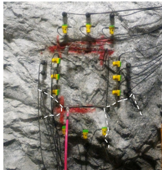
Fig. 17 Evidence of fractures at the end of the first test conducted in the 50/1 by-pass
