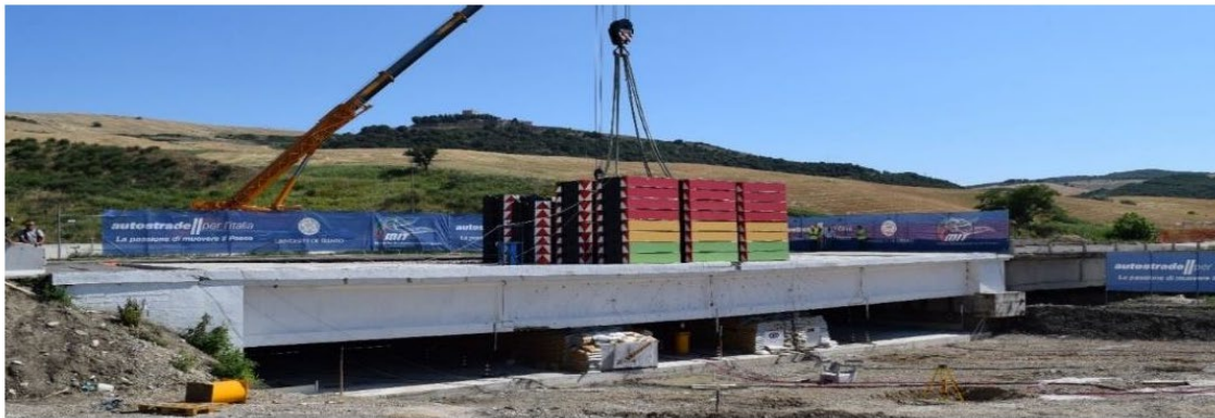
Figure 91: Picture of the Alveo Vecchio viaduct during the experimental test. Figure in [142].
