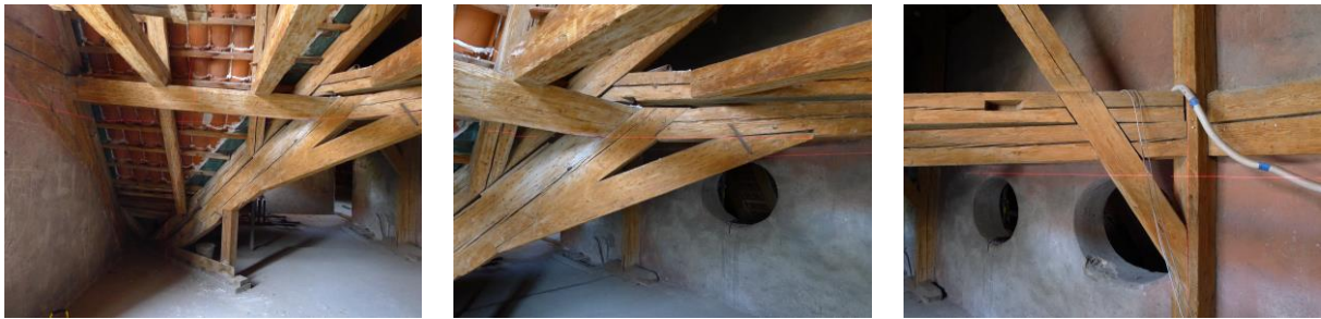
Figure 8 – The deformed frame of interest in the south part of the west wing
