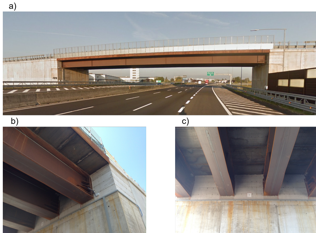
Figure 3.1: Integral abutment bridge which inspires the case study: (a) general view of the bridge, (b) detail of the integral connection at abutment-deck node, (c) detail of four welded I-shaped plate girders
