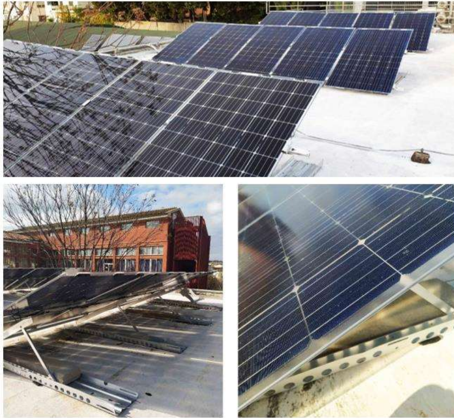
Figure 25. Photovoltaic system powering the SmartLAB
