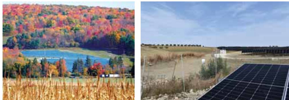
(a) Credits © Renantis Harford solar plant in New York—USA of 2.87 MW
