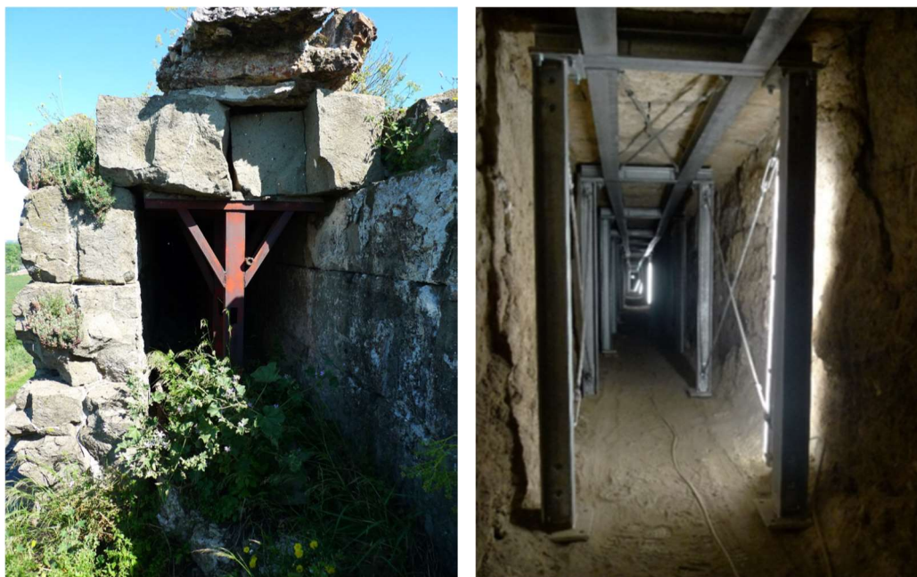
Figure 2: View of the hydraulic conduit in the end part of this section of the Claudius Aqueduct. The broken lintel is prop up by a metal support and in the upper part there is a residue of the Anius Novus upper structure. On the left, a recent anti-seismic intervention on an adjacent section.
