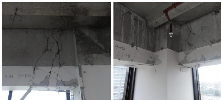
Fig. 1 Plastic hinges in the beams on the Precast 22-storey perimeter frame of the Price Waterhouse-Coopers PWC in Christchurch, New Zealand, after the 22 nd Feb 2011 Christchurch Earthquake (adapted from Kam et al. [1]).
