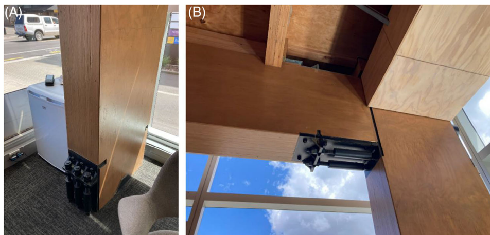
FIGURE 2 Example of (A) column-to-foundation connection and (B) beam-column connection with external damping devices, Young Hunter House, ‘Merritt Building’, Christchurch (NZ) (pictures courtesy of G. Formichetti).
