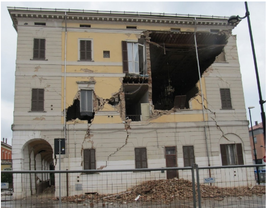
Fig. 1 Example of out-of-plane failure of URM wall connected to timber diaphragm during the 2012 Emilia, Italy earthquake
