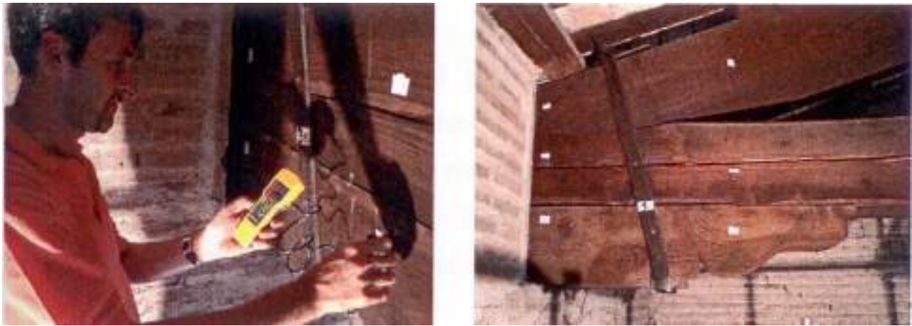
Fig. 62a. Moisture survey (left) and example of the coding assigned to the truss head with indication of the execution points (right). From P. Rocchi, C. Piccirilli, Manuale della Diagnostica , Edizioni Kappa, Roma 1999.
