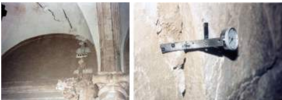
Fig. 43. San Bartolomé Parish Church. Structural consolidation. Foundation reinforcement through micropiles. Sewed of factories. Follow-up through instrumentation. Susana Mora. Tarazona de la Mancha, Albacete 2000.
