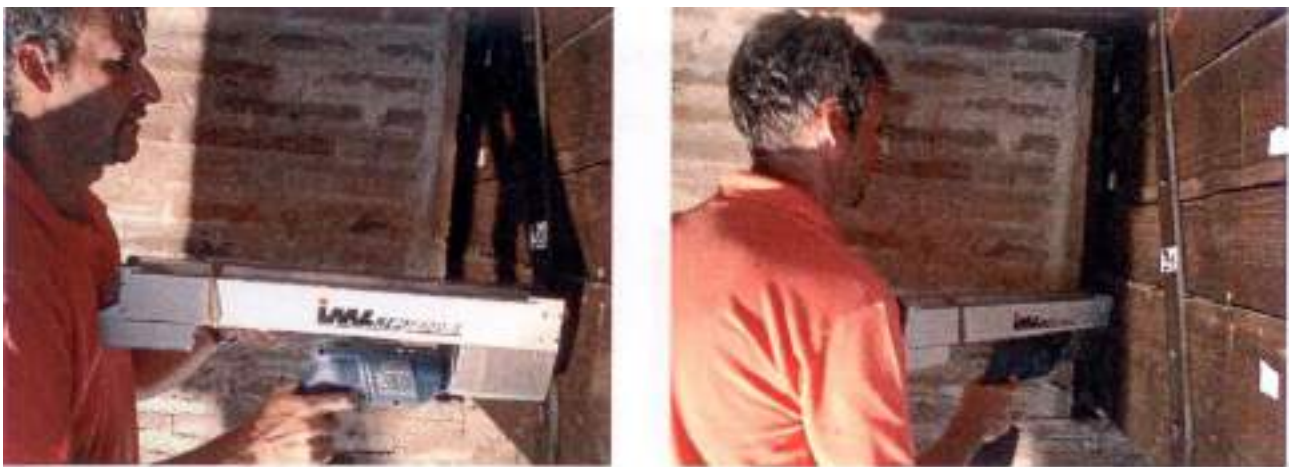
Fig. 62b. Perforations with resistograph in span (left) and in correspondence of the support (right). From P. Rocchi, C. Piccirilli, Manuale della Diagnostica , Edizioni Kappa, Roma 1999.
