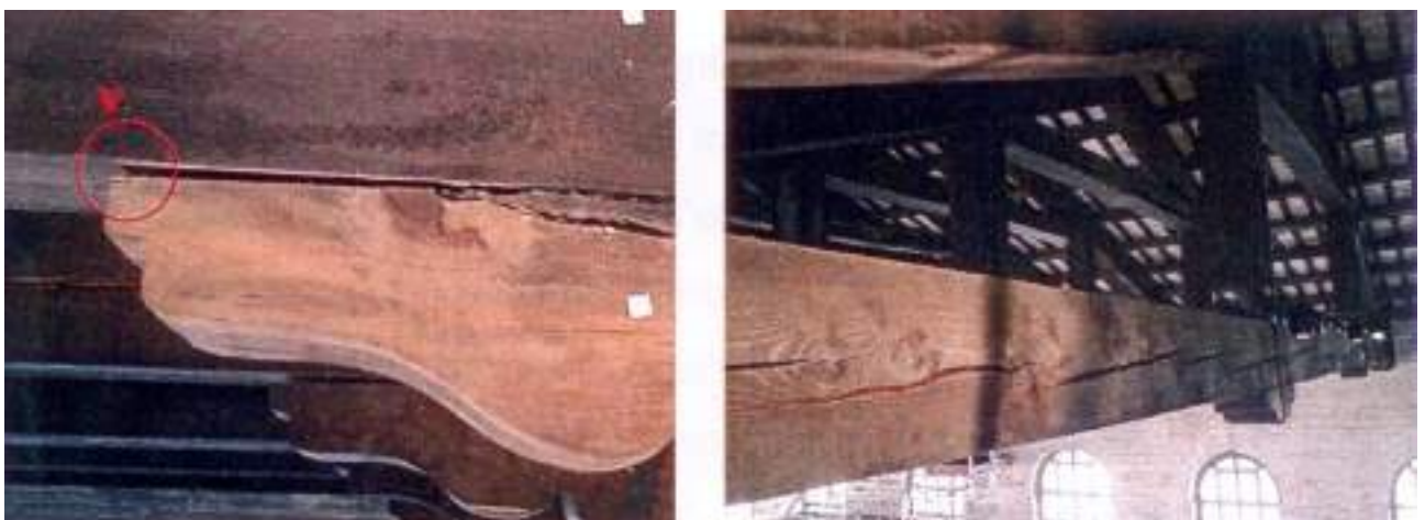
Fig. 60. Vertical deviation between bracket and tie-beam (left) and longitudinal fissures due to tie-beam shrinkage (right). From P. Rocchi, C. Piccirilli, Manuale della Diagnostica , Edizioni Kappa, Roma 1999.
