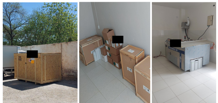
FIGURE 4. Pictures of stored new laboratory equipment. The boxes on the pictures were never opened several months after their delivery. The third picture shows equipment waiting for years to be completely installed.
