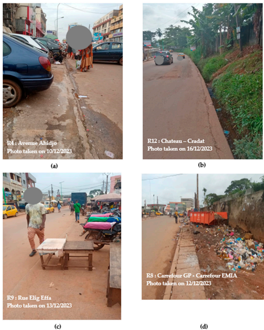
Figure 3. Predominant existing sidewalk condition on the road segments investigated: (a) existing sidewalk already in poor condition obstructed by cars and vendors; (b) total absence of sidewalk; (c) existing sidewalk obstructed by motorcycles and vendors. (d) lack of adequate sidewalk and obstruction of informal sidewalk (available space as well drainage).
