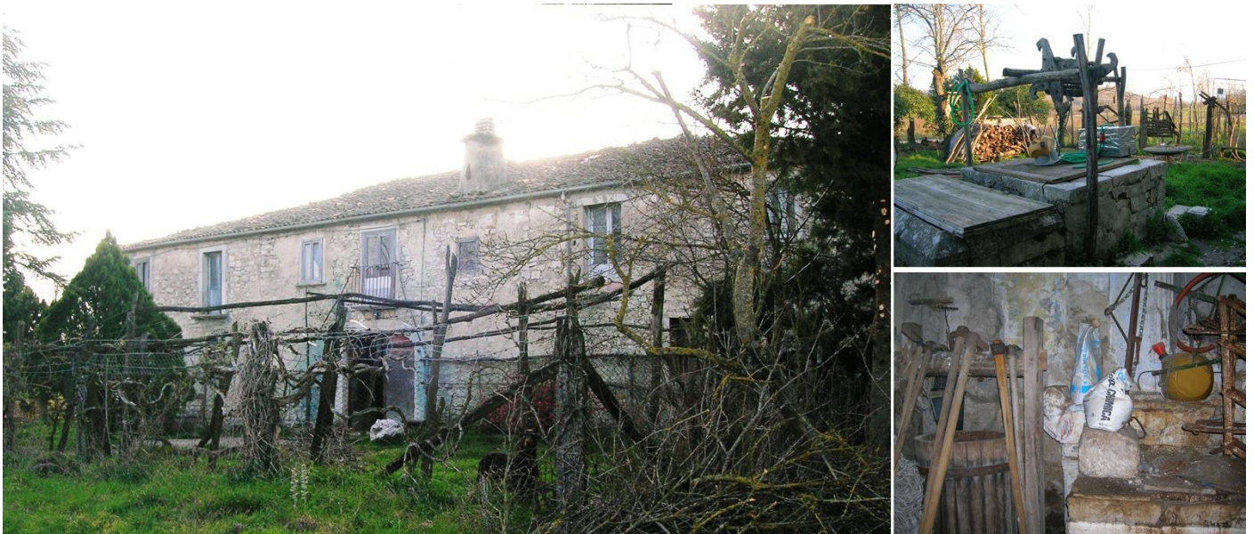
Fig. 8. Taverna of Sepino. It is a compact building, developed longitudinally, on two floors. It has wooden ceilings, and inside there is also a small chapel with some significant decorative elements. Unfortunately, there is no lack of collapses in this case either (photos of M. Vitiello).
