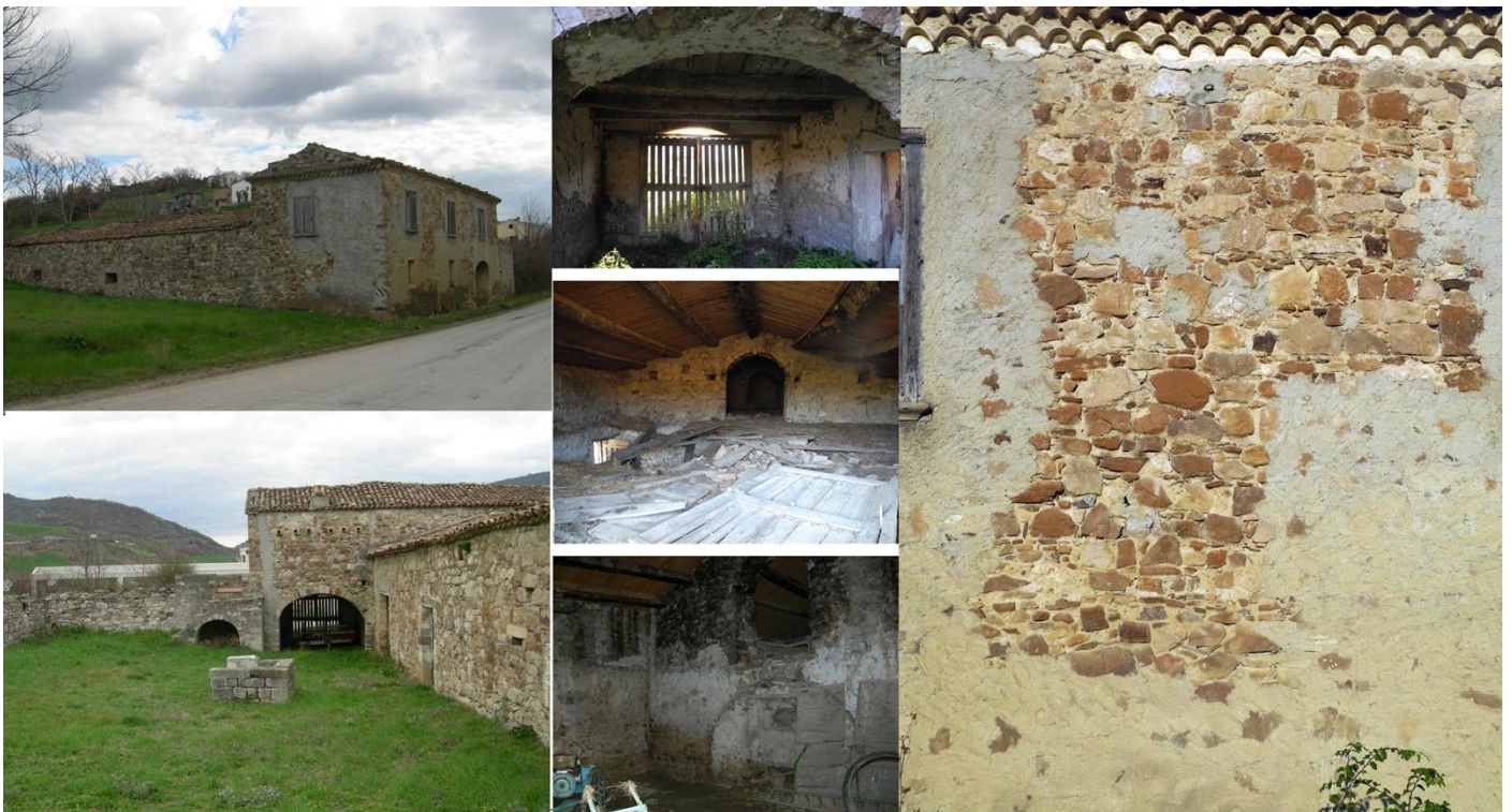
Fig. 9. Taverna of Trivento, View of the main front, inner courtyard, some interior rooms, and detail of the masonry (photos of M. Vitiello).
