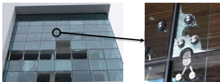
Figure 1. Example of damage in a PFGFS in a modern building located in Christchurch (left), and particular of the damage, due to tensile stress concentration, of the glass panel around the fixing zone (right), [Baird et al. 2011].
