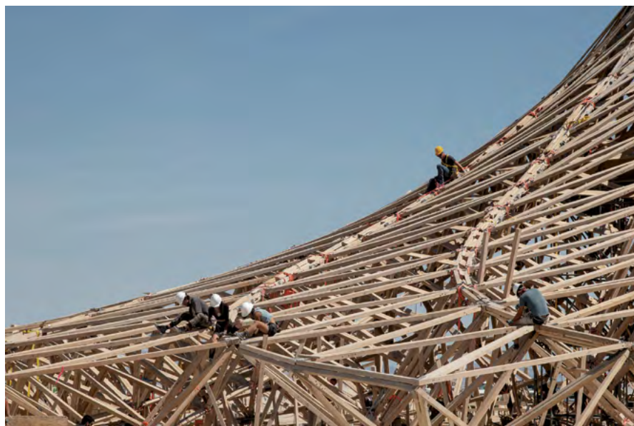
06. Costruzione partecipata del Temple. Burning Man, 2018 | Collective construction of the Temple. Burning Man, 2018. Angus McIntyre
