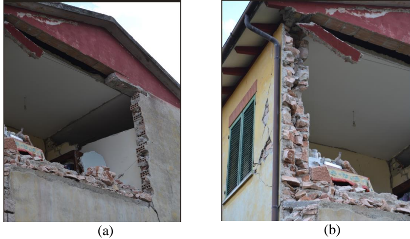
Figure 6: Details of the overturning mechanism of the North-West façade: (a) general view and vertically hollow block masonry; (b) concrete beam failure.
