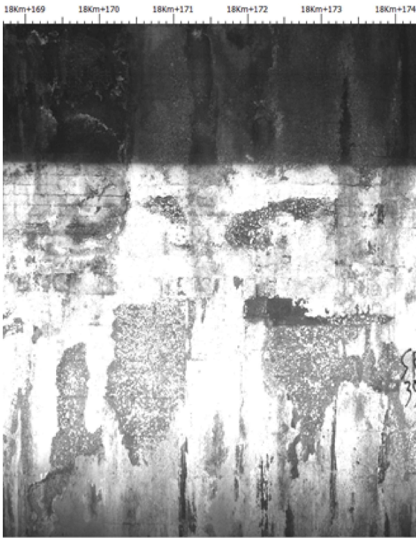
FIGURE 11. Detachment of concrete cover and exposure of the rebars (yellow area).
