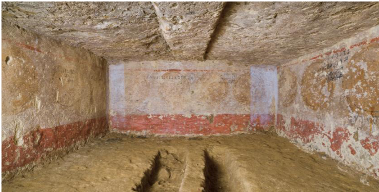
Figure 14. Burial chamber after the restoration. Two microbiological samples for each wall were studied.
