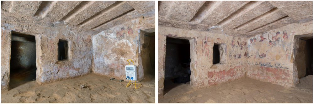
Figure 3. Tomba degli Scudi . South-east walls: before restoration (left) and after restoration (right).
