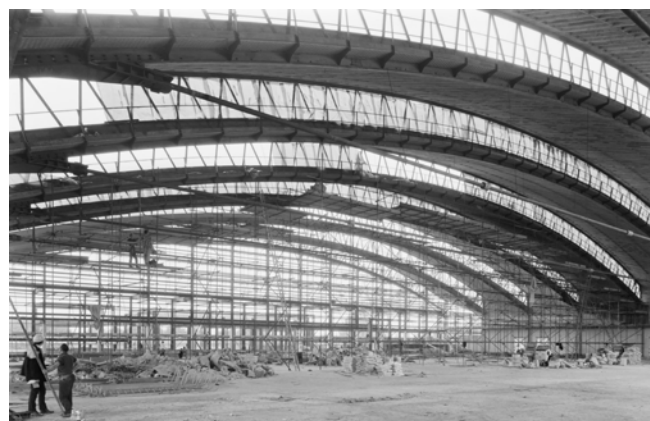
Figure 2. Application of the KS-shell to the Watney Mann Brewery, Isleworth, Hounslow, Greater London Authority (Historic England Archive, John Laing Photographic Collection, 1968).
