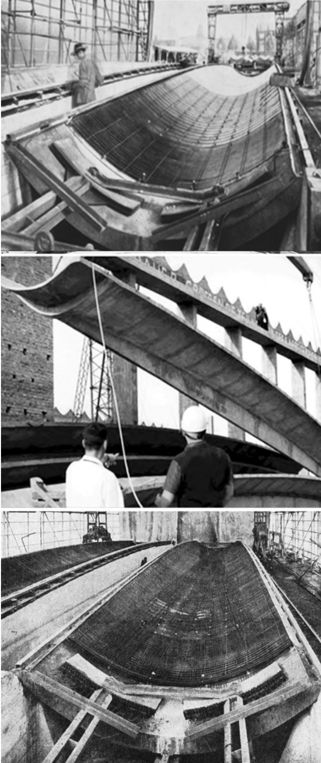
Figure 4. The three typologies of the Silberkuhl System for HP-shells roofing units (Silberkuhl, 1961a; Joedicke 1963).
