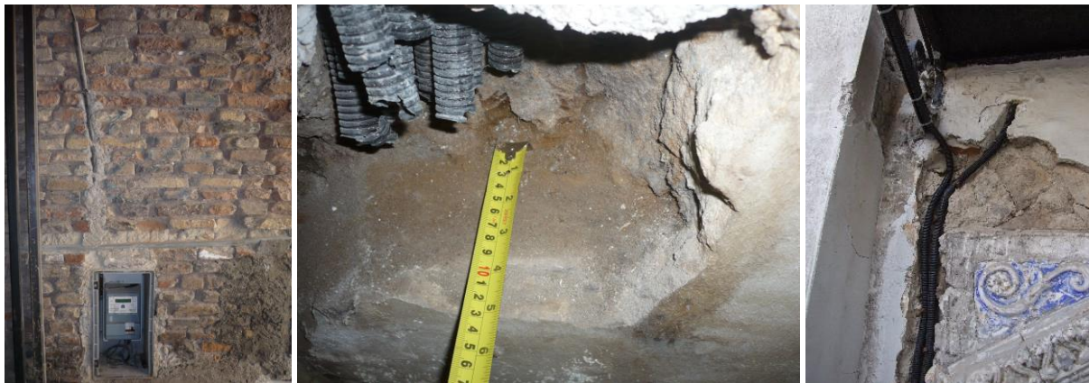
Figure 3: TBS placement on historic buildings with a high impact on load-bearing masonry structures
