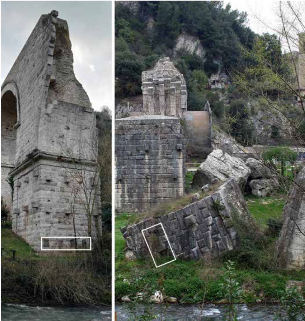
Figure 8. Holes in first and second pylon.
