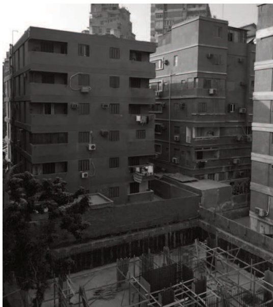
Fig. 8: Residential buildings from Modern Cairo "Mohandessin" and a construction site with traditional technologies (Author)
