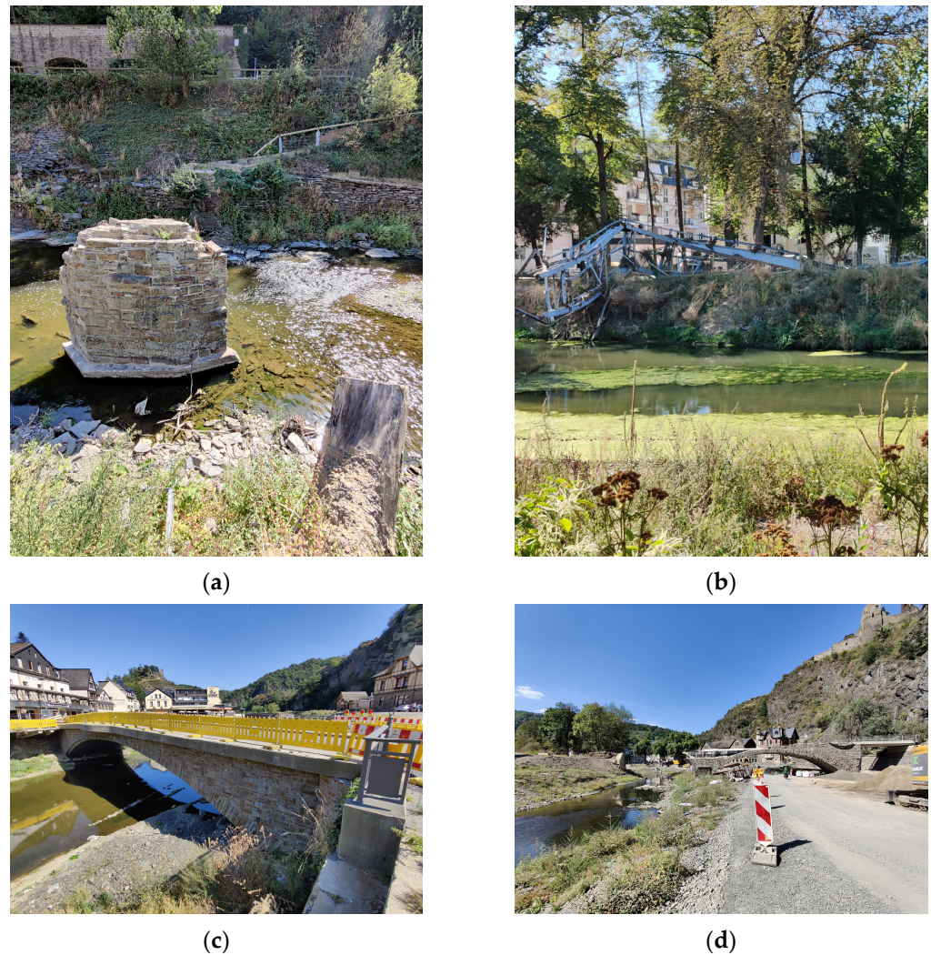
Figure 6. Surveyed overtopping mechanisms: (a) remaining pier of a dragged wooden deck; (b) girder of a dragged steel deck; (c) damaged railing due to overtopping; (d) combination of overtopping and scour, with the latter being responsible for triggering the failure. Pictures taken by the first author.
